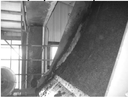
Primary Separation System (sloped screen)
